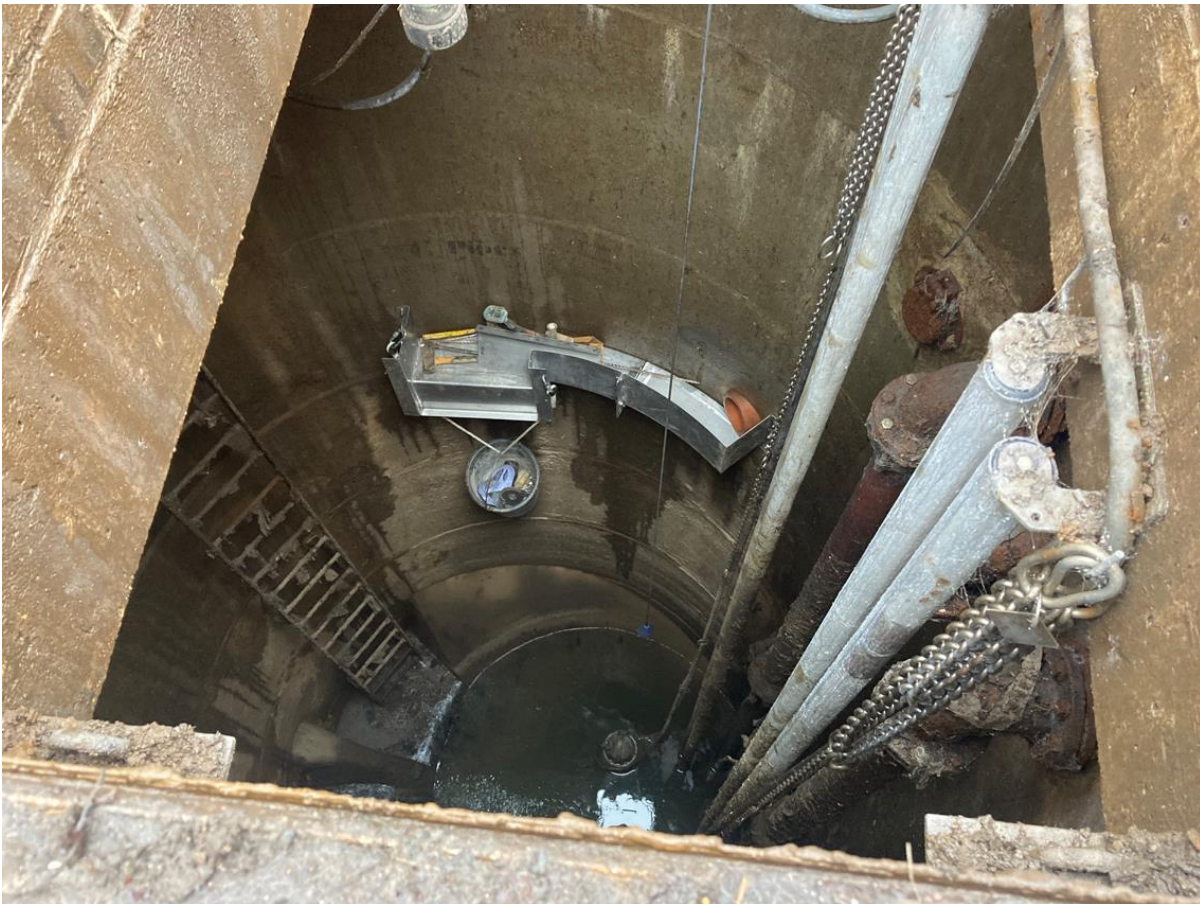
Ignore the hanging bucket! Outfall pipe is to the right in the new steel channel.
